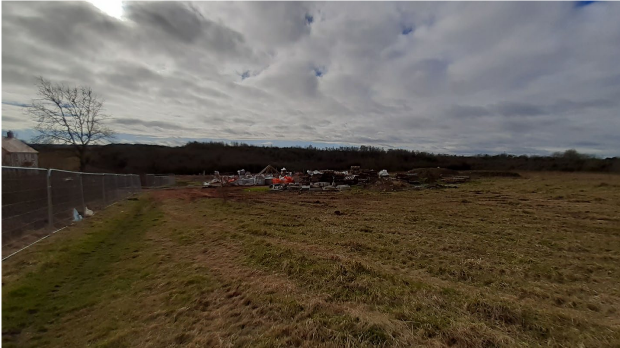
View south from north eastern part of site (with Phase D1 to left):
